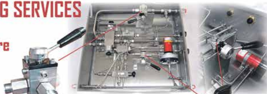
National Grid Slamshut Cabinet
